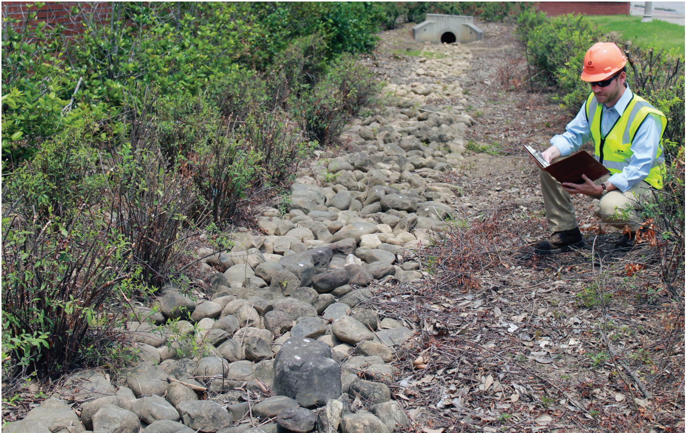
Nick Garner, Product Manager of Green Infrastructure for Oldcastle Infrastructure, inspects a traditional bioswale, a common piece of green infrastructure that utilizes biofiltration to remove stormwater pollutants.
