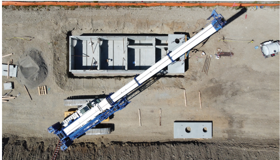
Installation of an Underground BioPod Biofiltration system from Oldcastle Infrastructure eliminated the need for multiple units and still met green infrastructure requirements in Fredrickson, Wash.
