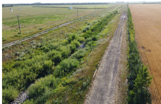
Vegetation establishment five months after installation (top) as well as channel performance five years after installation (bottom).
