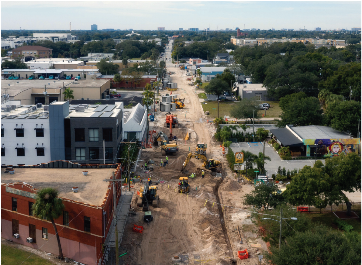
Installation of a multi-solution stormwater management system manufactured by Oldcastle Infrastructure for the Cypress Street area of Tampa, Fla.
