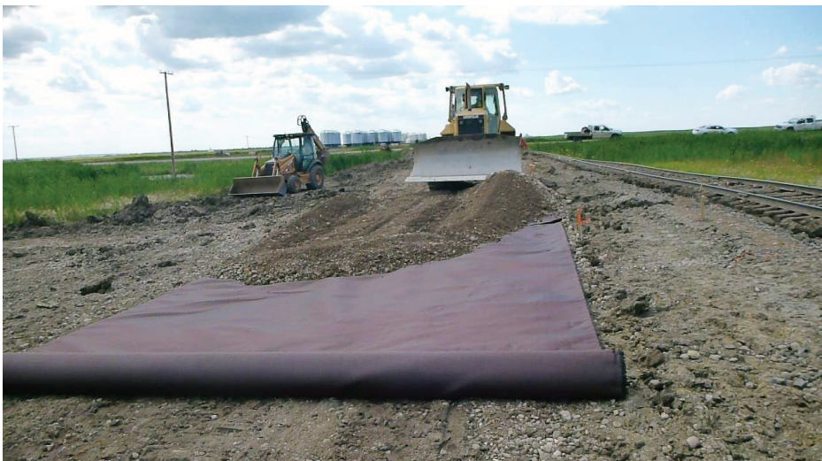
Incorporating MIRAFLI RS580i geosynthetics as part of the Rosetown rehabilitation, CN was able to successfully repair a track section that had been rehabilitated 20 times in the previous five years.
