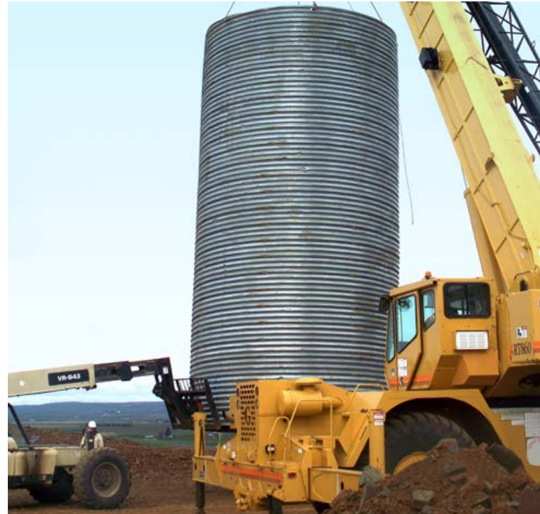
HEL-COR® is an integral part of the design of the turbine foundation.
