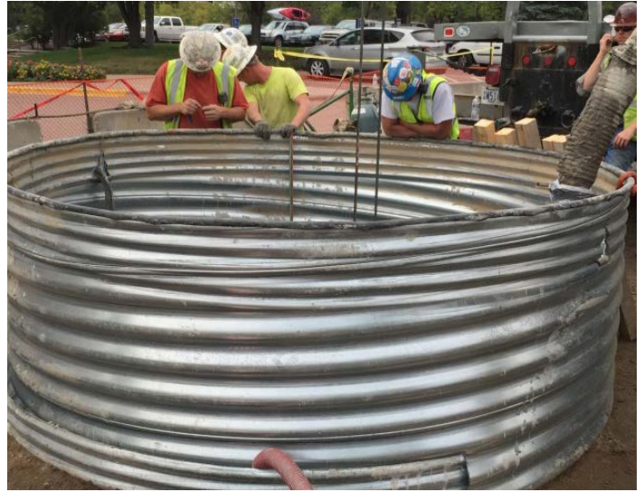
Vertical access shafts can be used to safely access utilities below ground.
