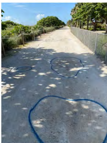
Figure 15- 4C Potholes Photo 1
