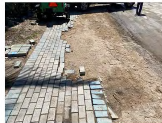
Figure 68- 9M 88 ST Damages Photo 1
