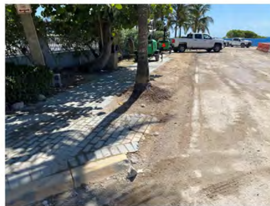
Figure 67- 9L 88 ST Damages Photo 1
