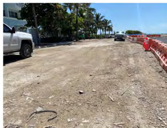
Figure 65- 9J 88 ST Damages Photo 1
