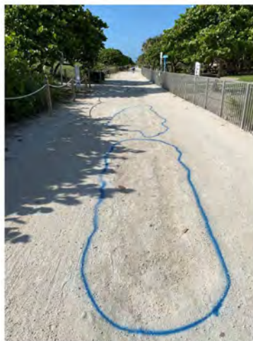
Figure 14- 4B Potholes Photo 1
