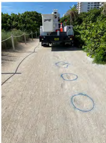
Figure 13- 4A Potholes Photo 1
