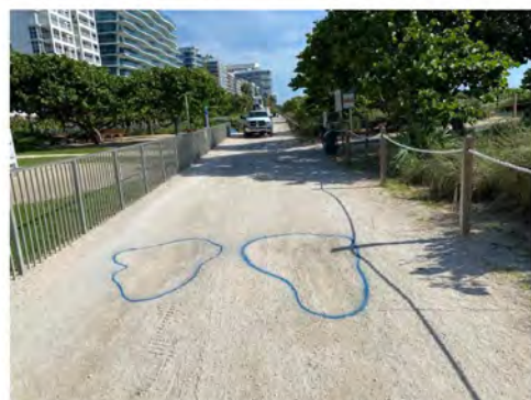
Figure 16- 4C Potholes Photo 2
