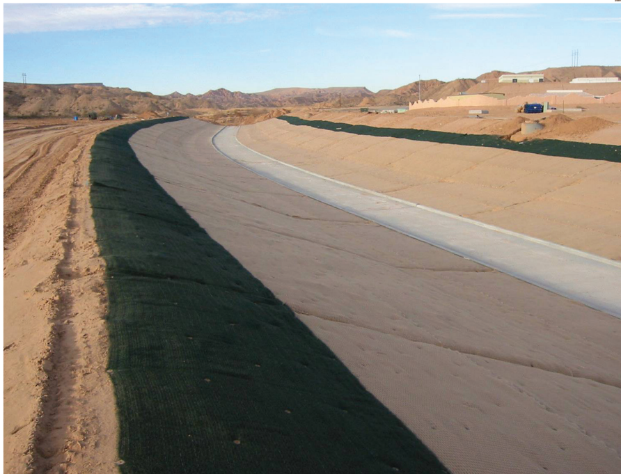
Abbott Wash Channel was installed in 2002 (left). A photo shows the Abbott Wash Channel's performance in February 2021 (right).
